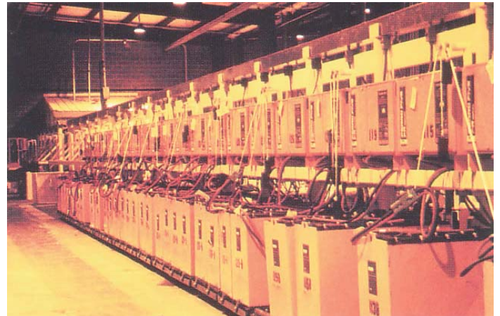
To obtain a high level of forklift usage with minimum disruptions Bi-Lo installed a new battery charging room with 60 state-of-the-art chargers, furnished by C & D Charter Power Systems.
